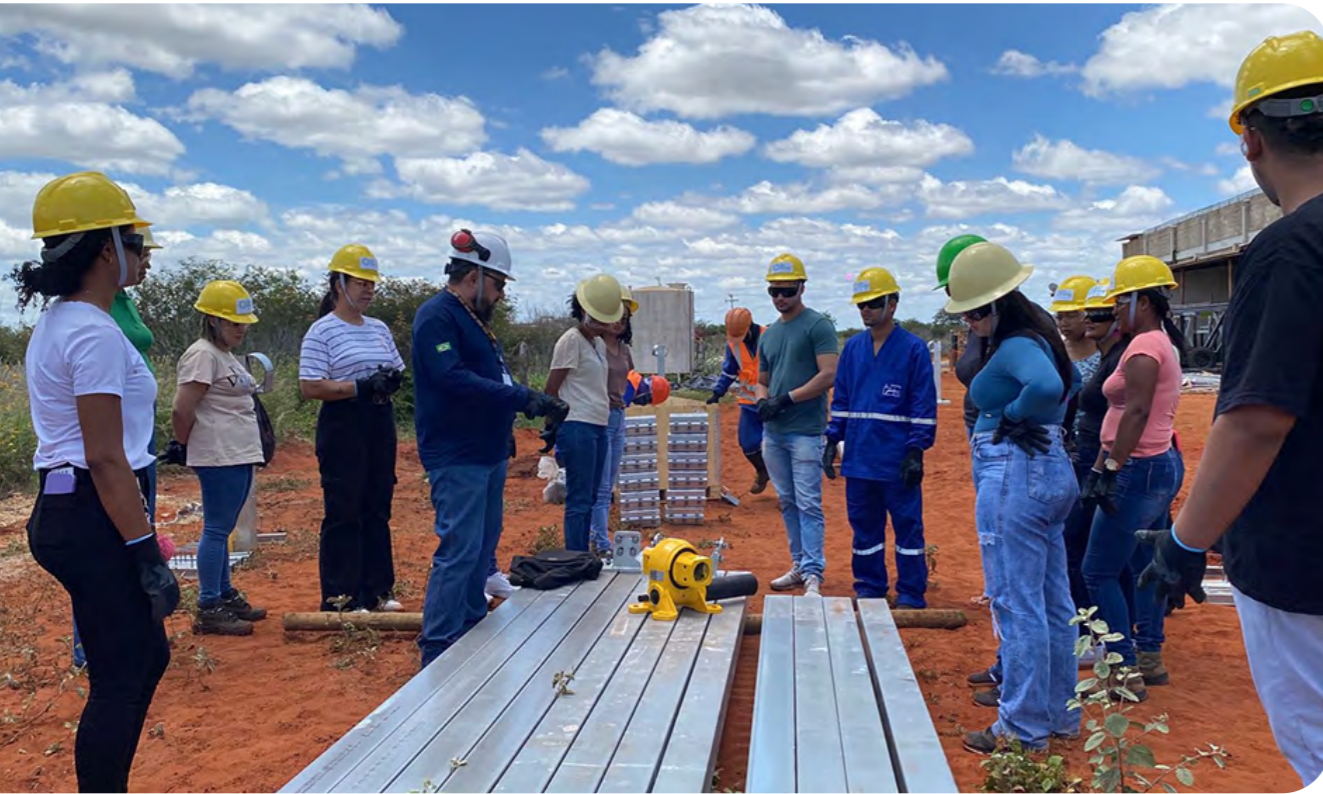
Practical class of the tracker assembly course held at the construction site of the Serra da Babilônia Solar Complex.
